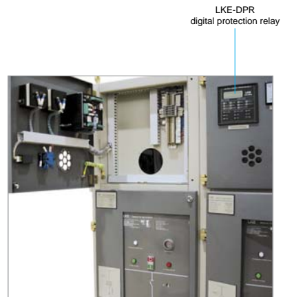
Low voltage compartment
